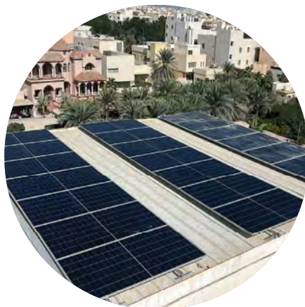
25 kWp on-grid rooftop solar PV system for private residence.
