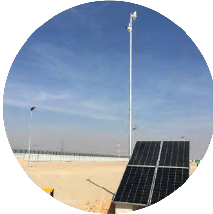
20 kWp off-grid ground-mounted solar system.
