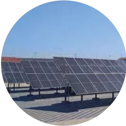
165 kWp on-grid ground-mounted solar PV system.
