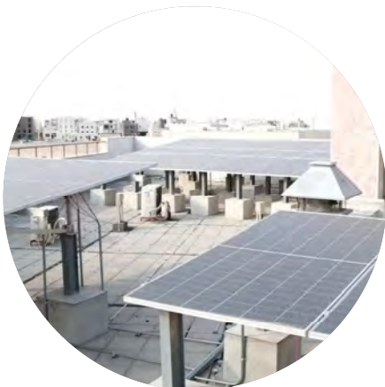
20 kWp on-grid rooftop solar PV system.
