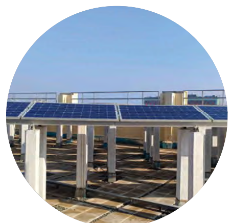
Smart Building solar systems 65 kWp roof-mounted on-grid solar PV system.
